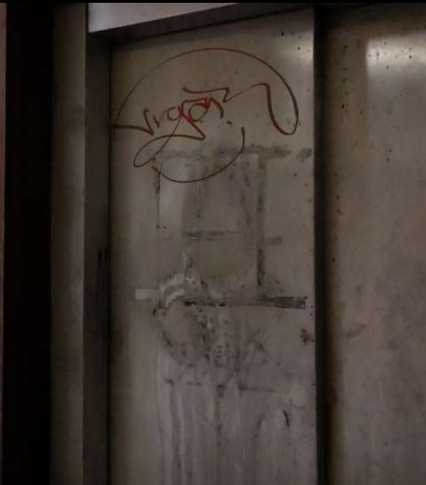
Lift doors. Lifts not working on day of visit, so no interior photos.
