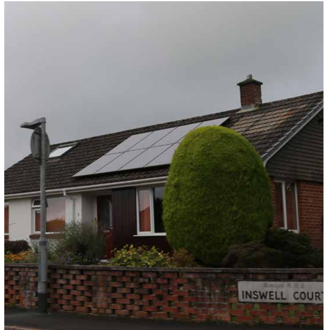
Figure 88: - A property with PV installed.
